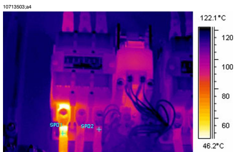
Figure 21.9 An infrared image of indoor electrical equipment (2)
