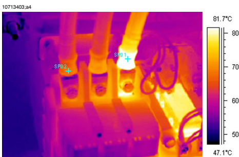
Figure 21.8 An infrared image of indoor electrical equipment (1)
