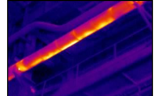
Monitoring of cables
