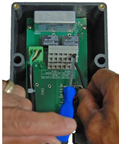
Figure 6: Electrical Connections on Terminal Block (P1)
