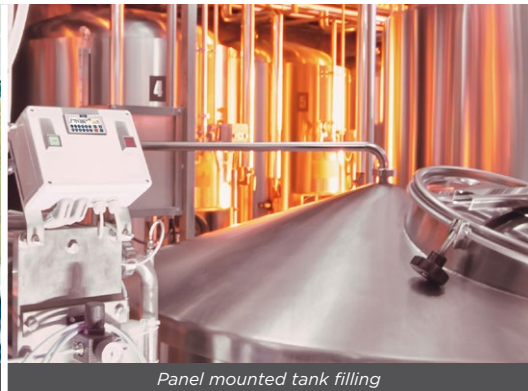
Panel mounted tank filling
