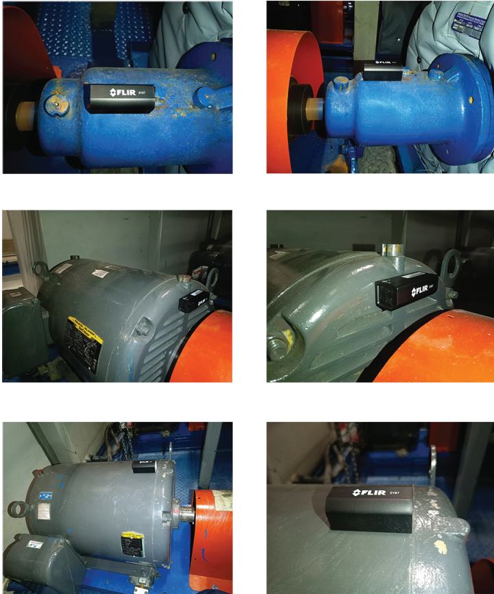
Figure 6.2 SV87 Sensors shown mounted on machinery.
