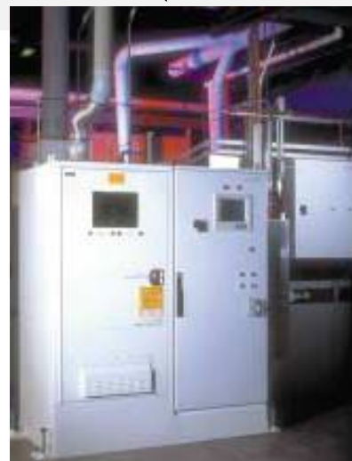
Gas Delivery Cabinet
