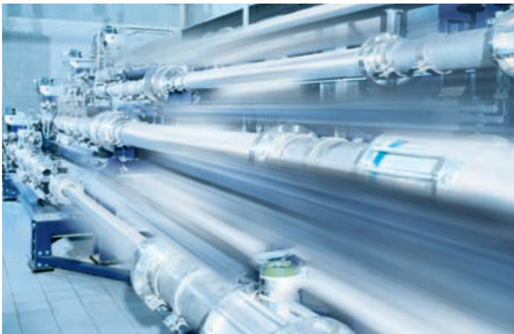
Calibration Facility of Rota Yokogawa, 79664 Wehr, Rheinstr. 8, Germany
