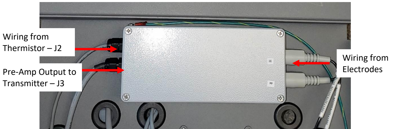
Figure 10. Pre-amplifier located behind the wet panel.
