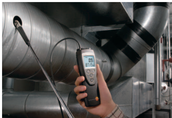
testo 416 monitoring the volume flow of exhaust air
