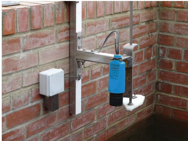
Figure 3-6. Open weir chamber arrangement with Rosemount Head Verification Device
