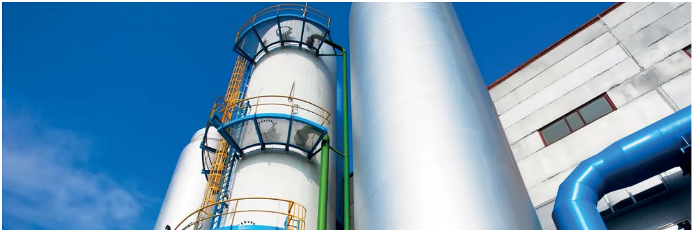
Air Separation Plant
