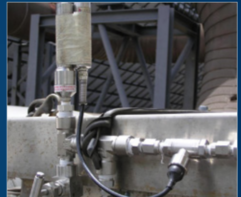
Orifice Plate Monitoring
