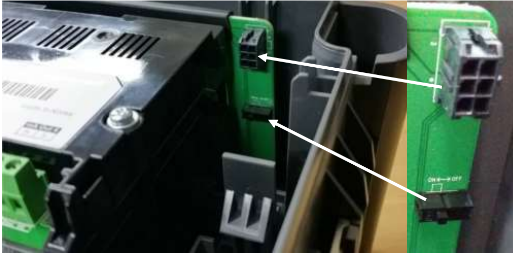
Figure 52. Battery On/Off Switch and Battery Connector
