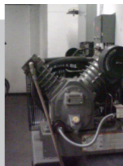
Air Compressor – Full Visible
