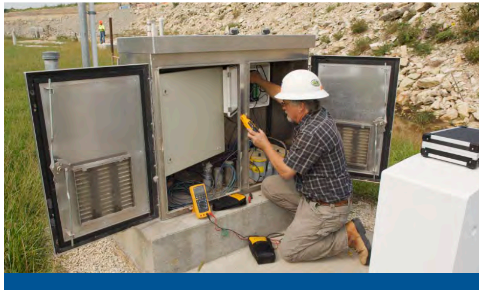
Bob Frazey works in one of the sensor service panels that lay across the base of the dam. These service panels are all low voltage panels that house ground swell sensor communications and support systems. He uses the Fluke 189 DMM to check the 12 V dc battery charging system that comes from a nearby solar panel. He also uses the Fluke 771 Milliamp Process Clamp Meter to check the 4 mA to 20 mA signal from the pressure sensors and transducers.
