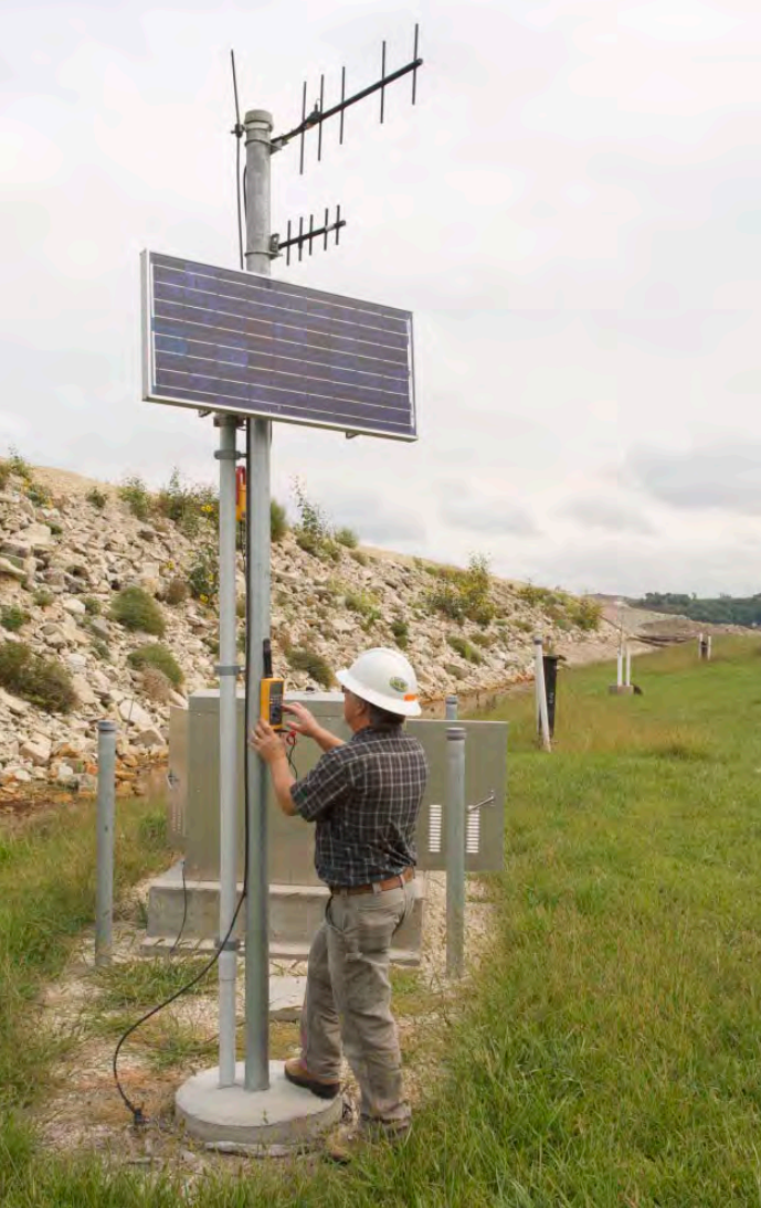
The Fluke 1630 is also used to check the grounding wire on the mast of the radio antenna and solar charging panel. Frazey also uses the Fluke 189 DMM with a Fluke i410 current clamp to look at the current output of the solar panel to the battery charger inside the service panel.
