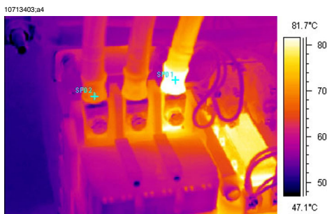
Figure 25.8 An infrared image of indoor electrical equipment (1).
