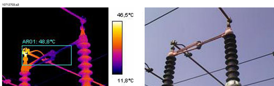
Figure 25.1 An infrared and a visual image of a power line isolator
