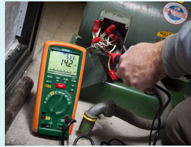
Insulation test on pump motor
