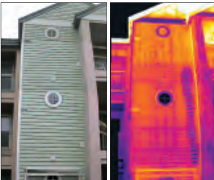
The thermogram of this vinyl-sided 3-floor apartment building clearly shows the path of a serious leak, completely hidden within the wall, from a washing machine on the third floor.
