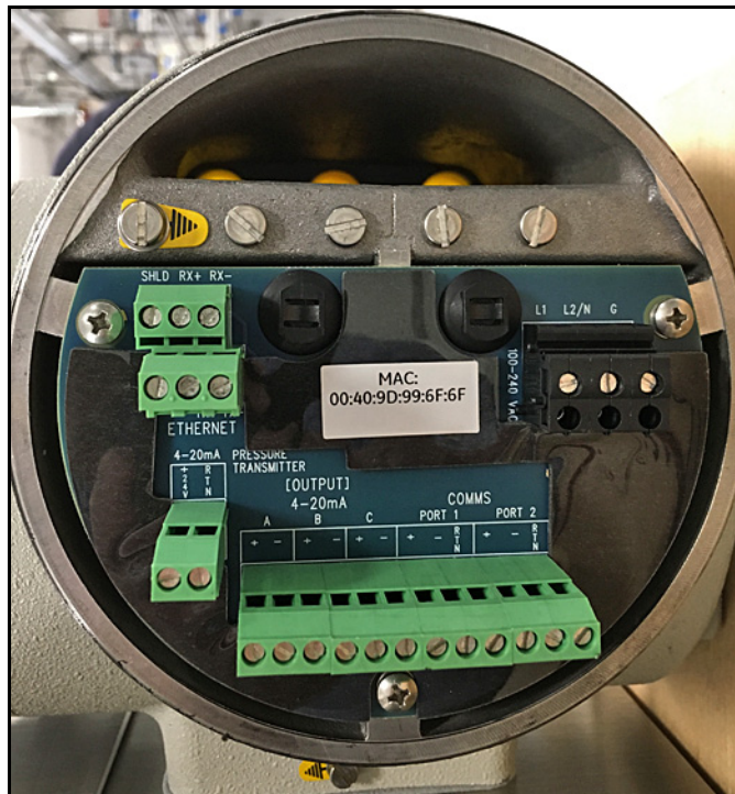
Figure 25: Wiring Terminal Blocks
