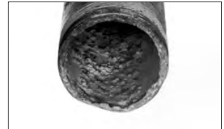
Figure CG-10. Oxygen in the system speeds corrosion (oxidation) of pipes, causing pitting such as shown here.
