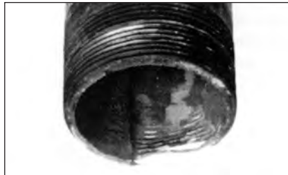
Figure CG-9. CO 2 gas combines with condensate allowed to cool below steam temperature to form carbonic acid, which corrodes pipes and heat transfer units. Note groove eaten away in the pipe illustrated.
