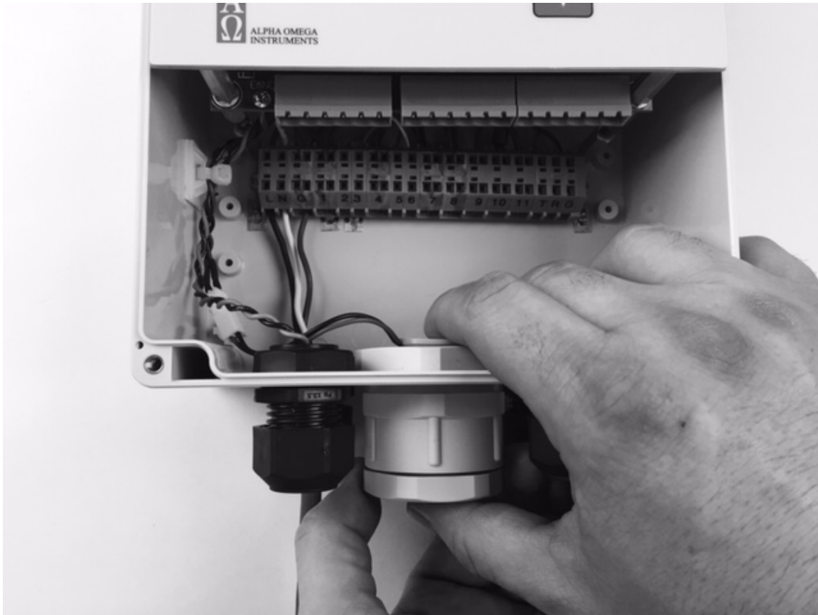
Figure 7 - Local Oxygen Sensor Installation
